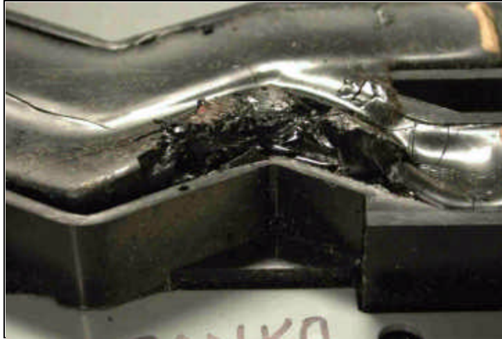
FIGURE 3 - OVERHEATING AT THE CONTACT BETWEEN THE BUSSBAR AND THE STAB SOCKET ASSEMBLY CAUSED THIS DAMAGE TO THE INSULATION.
